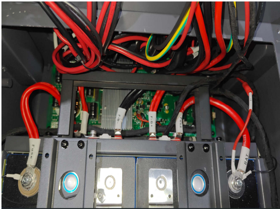
Internal view 3 of battery system
